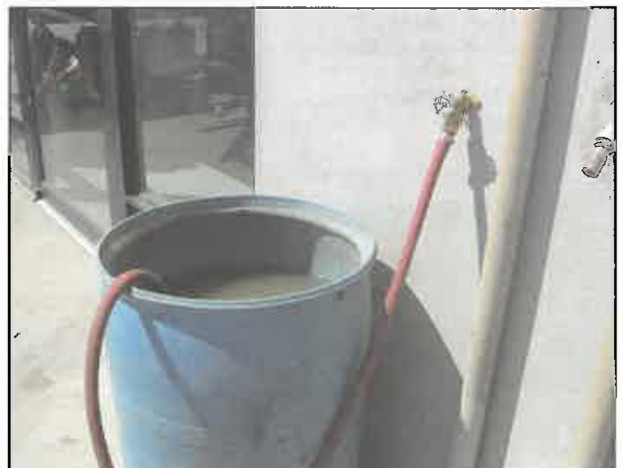
Hose submerged in a barrel of water is a cross-connection hazard.
